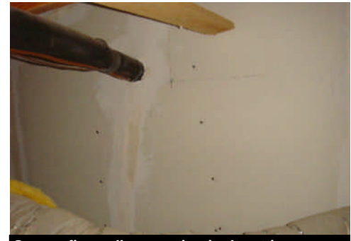
Garage fire wall separation in the attic.
