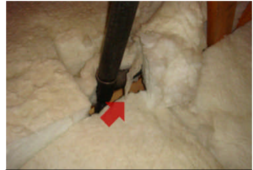
Void, on top of pipe and framing.
