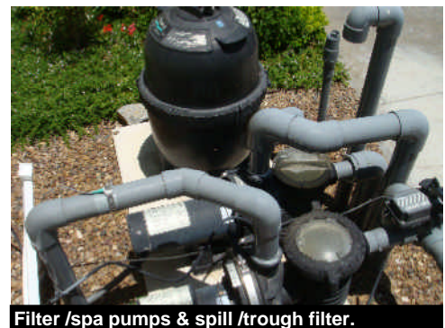
Filter /spa pumps & spill /trough filter.
