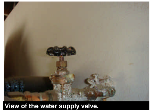
View of the water supply valve.
