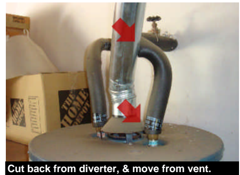
Cut back from diverter, & move from vent.
